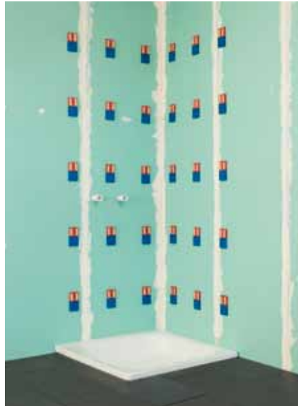
Installing a rear shower wall by means of the key and lock principle
