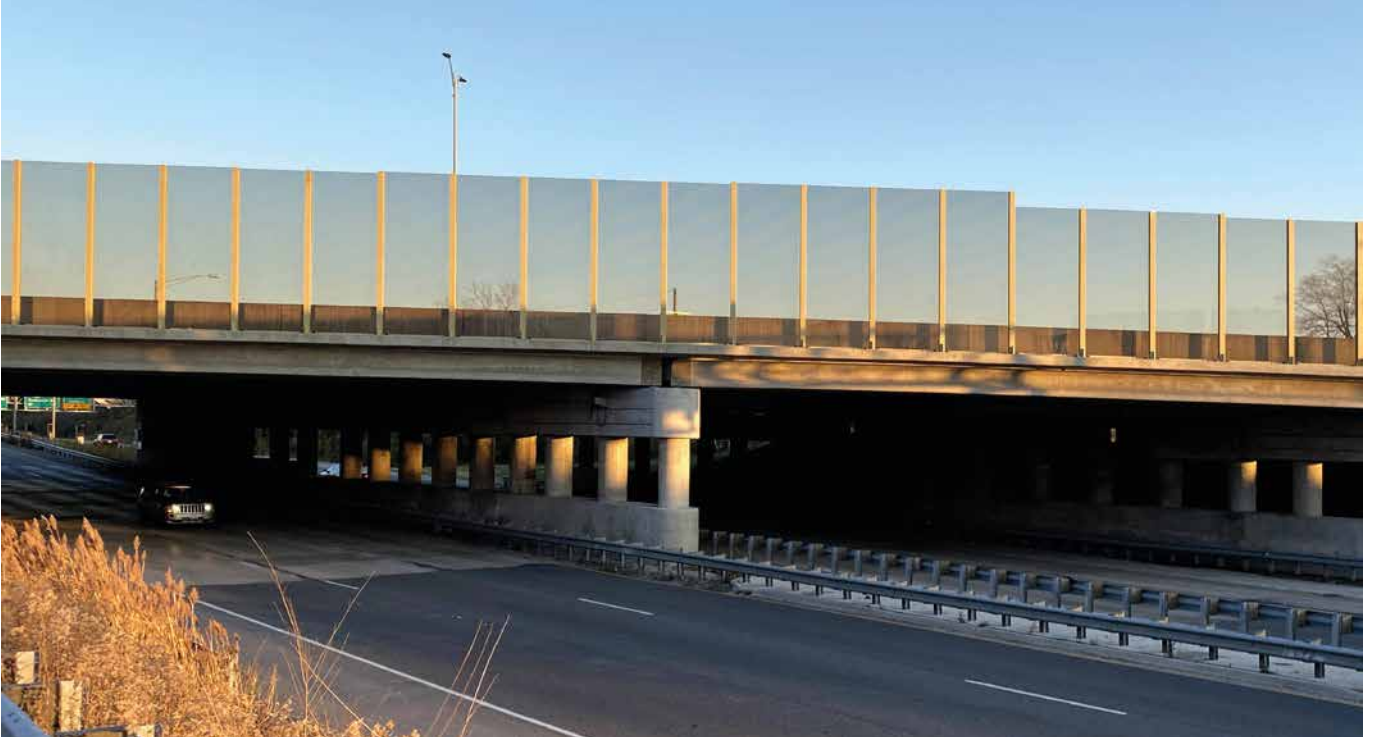
Noise barrier, I-88 over Roosevelt Road and IL-38 in Elmhurst, IL ACRYLITE® Soundstop GS CC Smoky Brown
