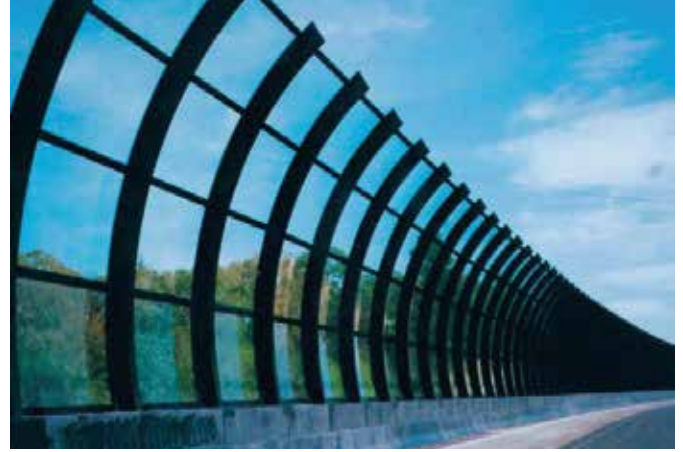
Noise barrier, M5, Melbourne PLEXIGLAS® Soundstop John Holland
