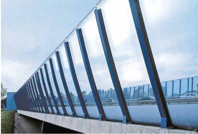
Noise barrier, Velperbroek PLEXIGLAS® Soundstop XT Combinatie Heijmans-Strukton
