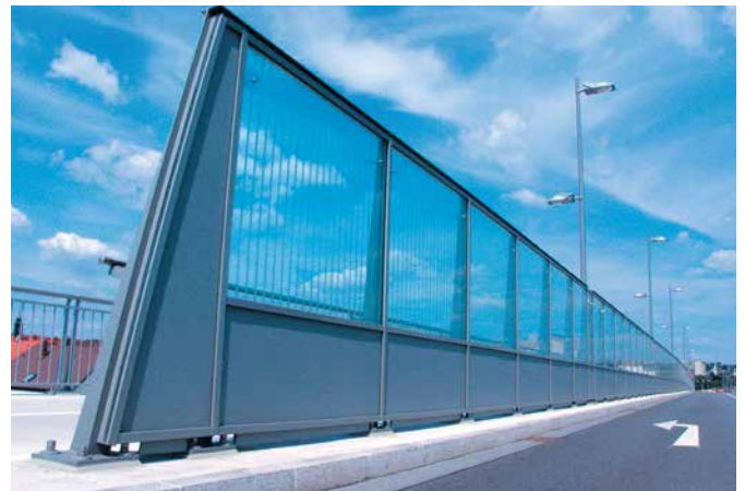
Noise barrier, Nibelungenbrücke, Regensburg Lower part made of PLEXIGLAS® Soundstop NT Fa. Markus Kaiser
