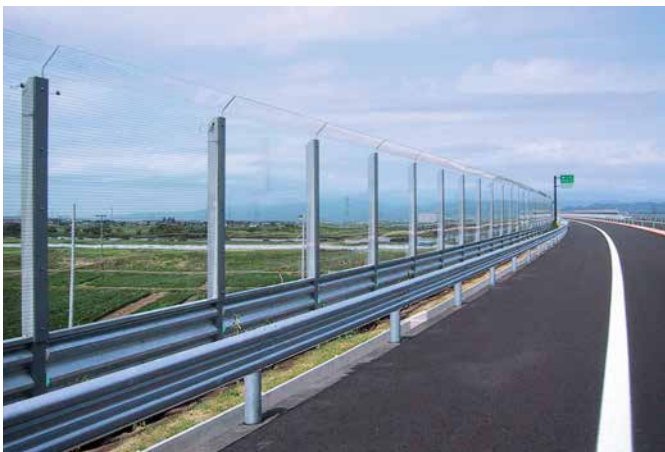
Noise barrier, Highway Tsuruoka PLEXIGLAS® Soundstop GS CC Tsuruoka
