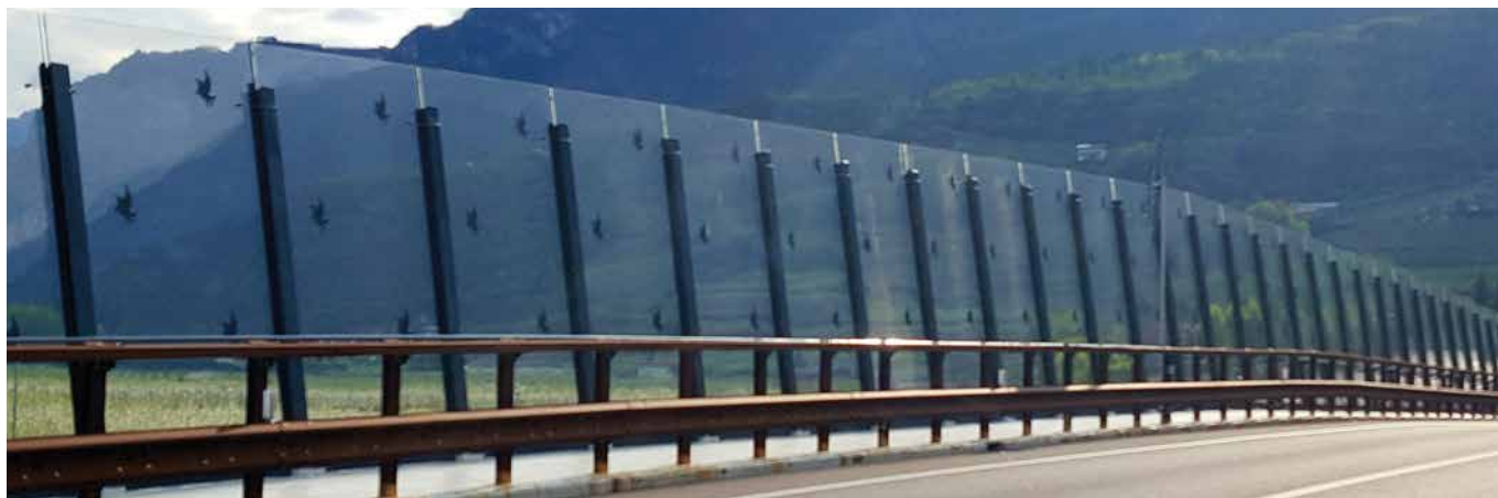
Noise barrier, Highway Trento Sud Flyover PLEXIGLAS® Soundstop GS CC 20 mm, Clear Trento Sud Flyover
