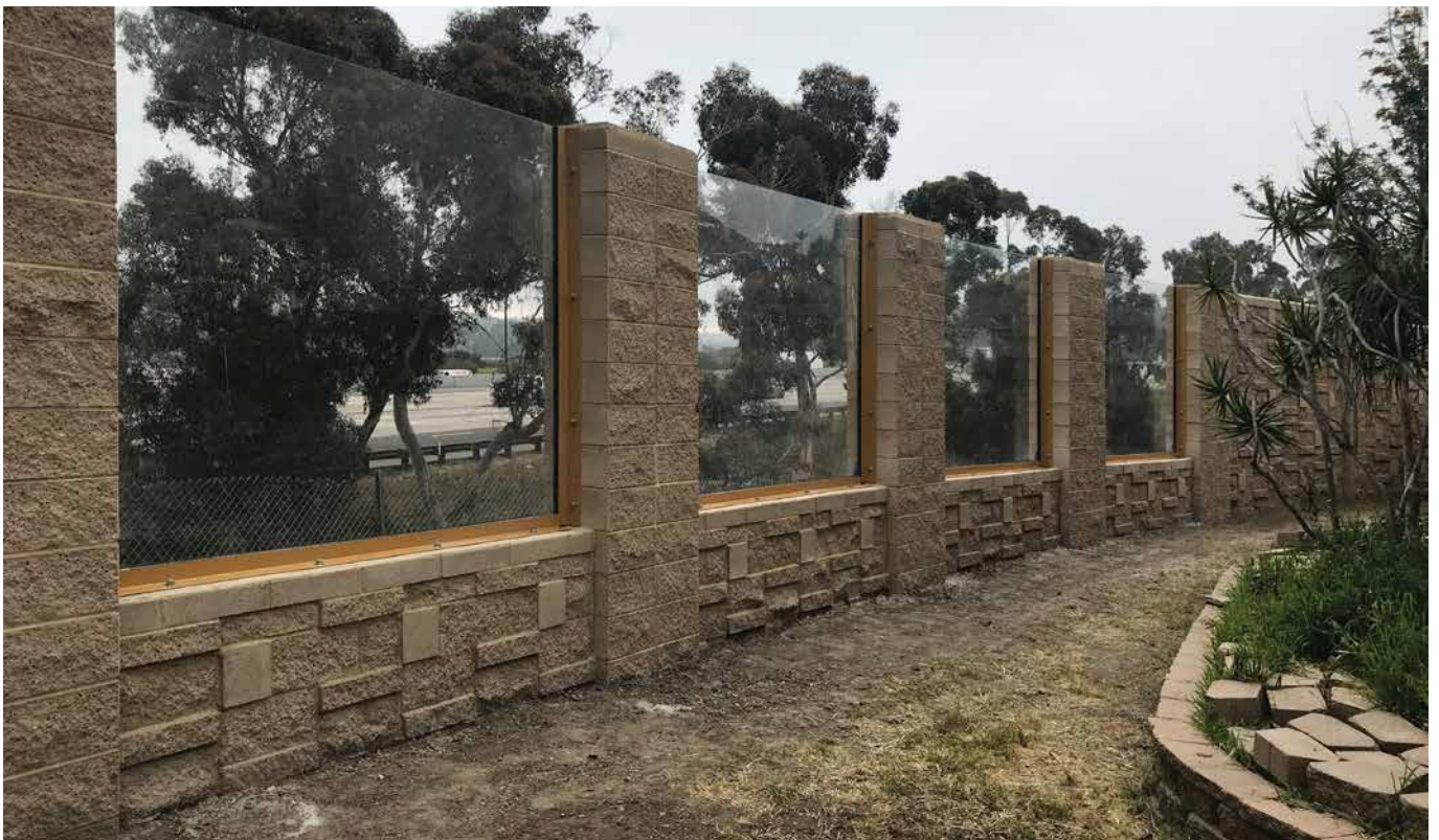
Noise barrier, near Telegraph Canyon Road off the I-805 Freeway in Chula Vista, CA ACRYLITE® Soundstop
