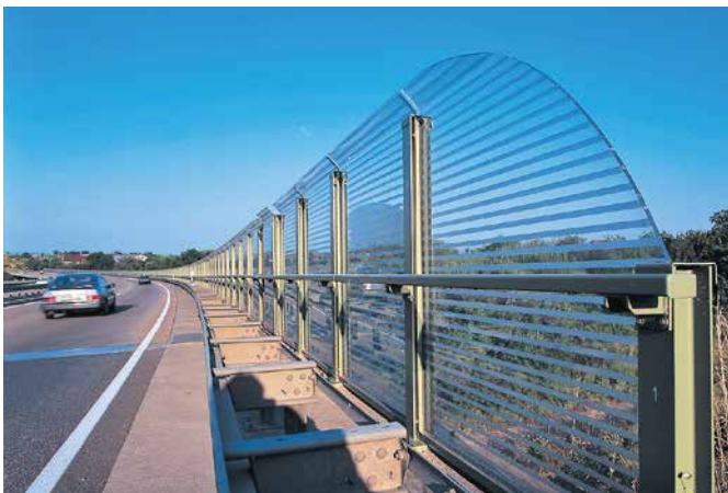
Noise barrier, Eltville PLEXIGLAS® Soundstop XT
